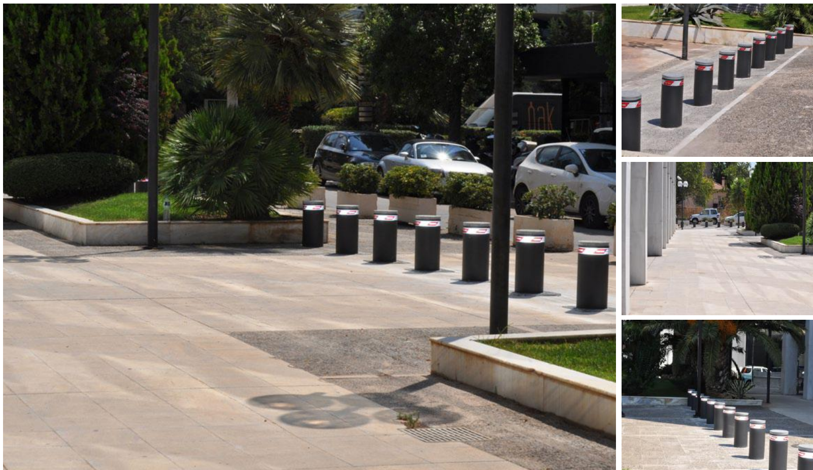
Installation with automatic rising bollards 275/P 600A
