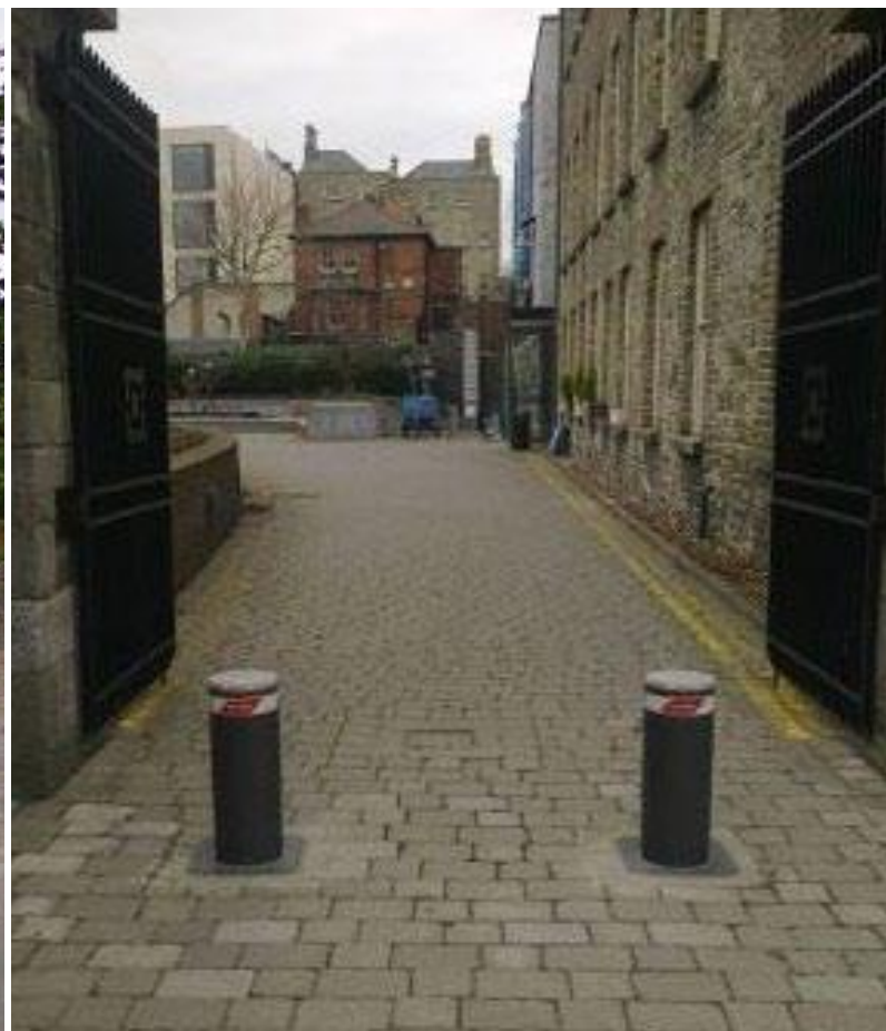
Installation with automatic rising bollards 275/P 600A
