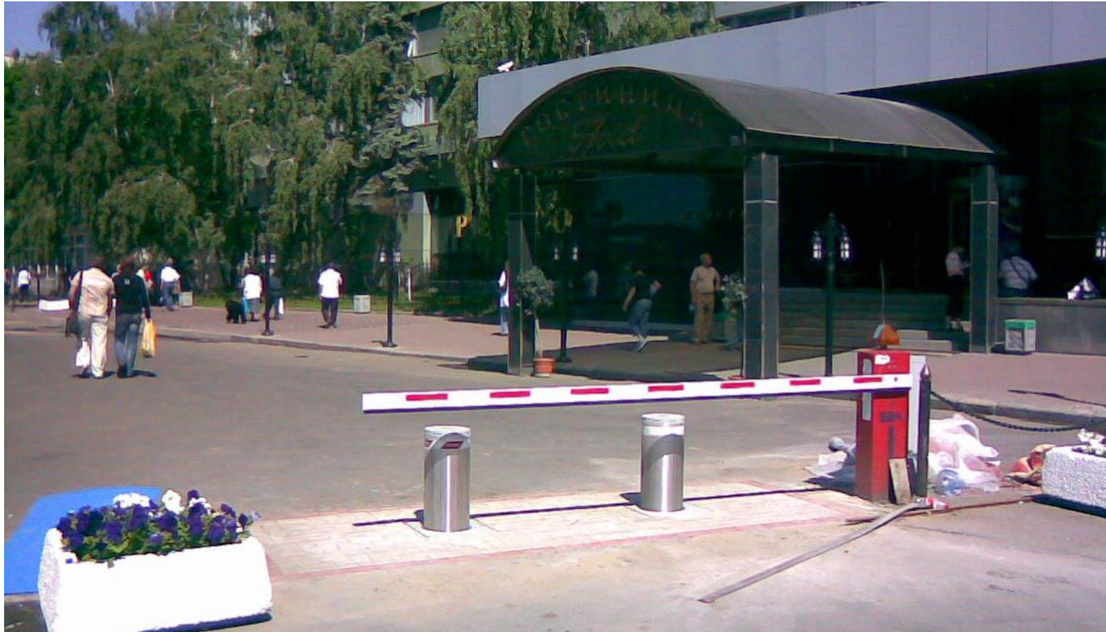
Installation with automatic rising bollards 275/P 800A
