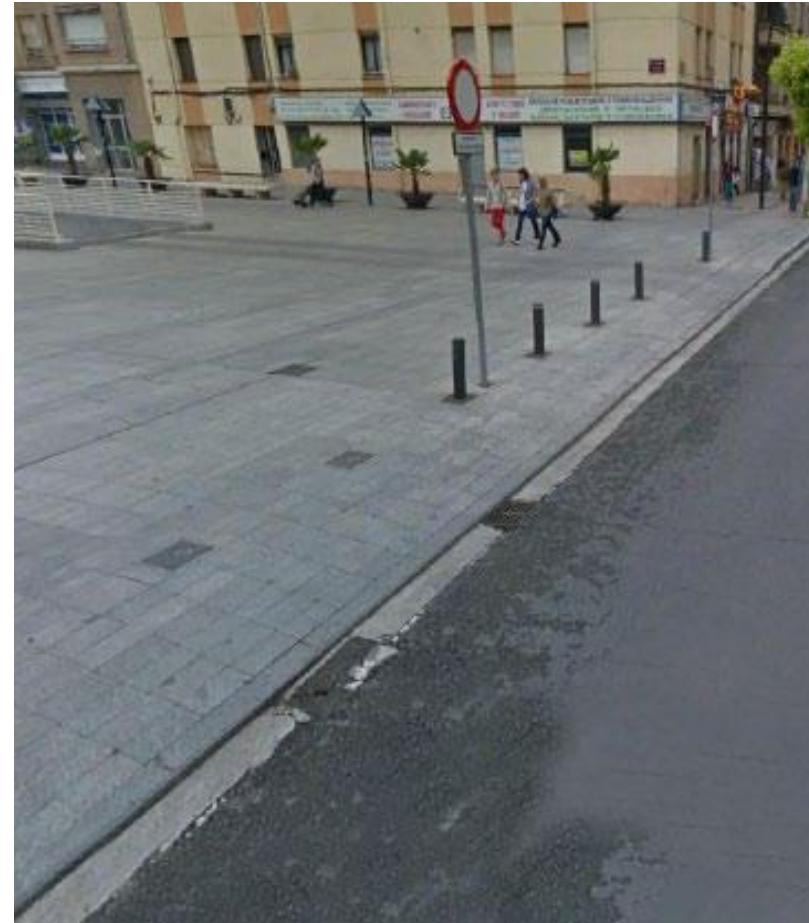
Installation with automatic rising bollards 127/P 600A
