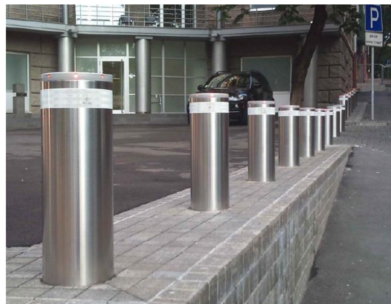
Installation with automatic rising bollards 275/P 600A
